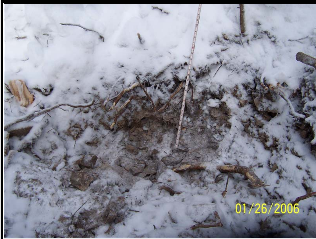
Partially backfilled test pit at A1 NA (north anchor), prior to reexcavation and drilling.
