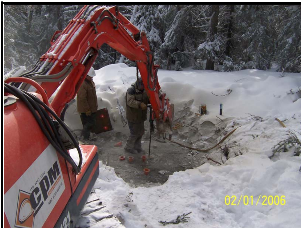
Manually operated jack hammer drilling at A1 SA (south anchor). Back hoe is being used to assist operator with down pressure on jack hammer.
